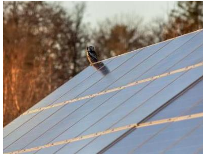
PV modules on roof
